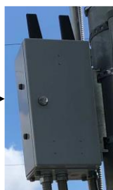
SPaT information roadside unit (newly installed) • Controller-based method • LTE connection
