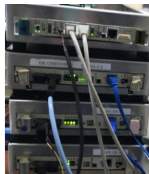
Terminal control unit
