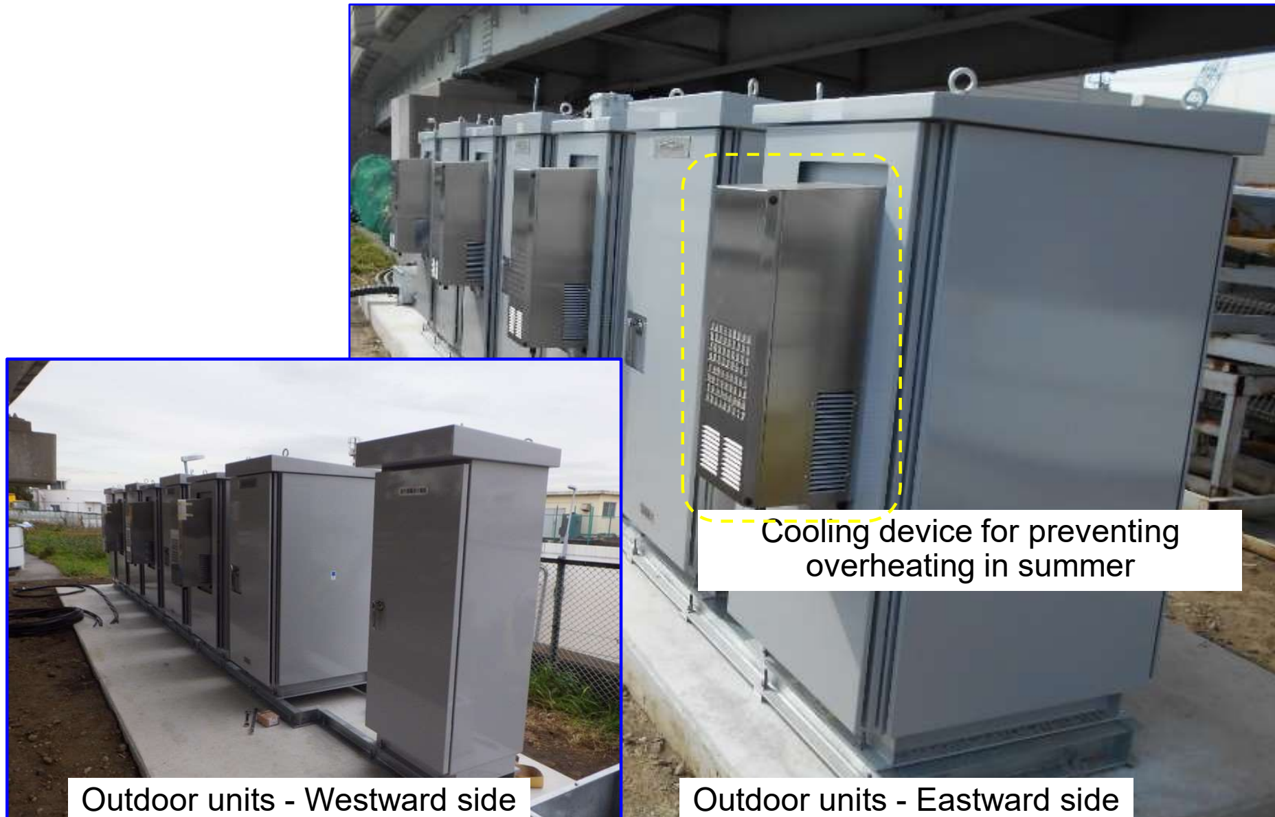
Figure 3-6 Appearance of outdoor units that house ETC gate passing support information provision management servers and processing roadside units of individual sensor manufacturers
