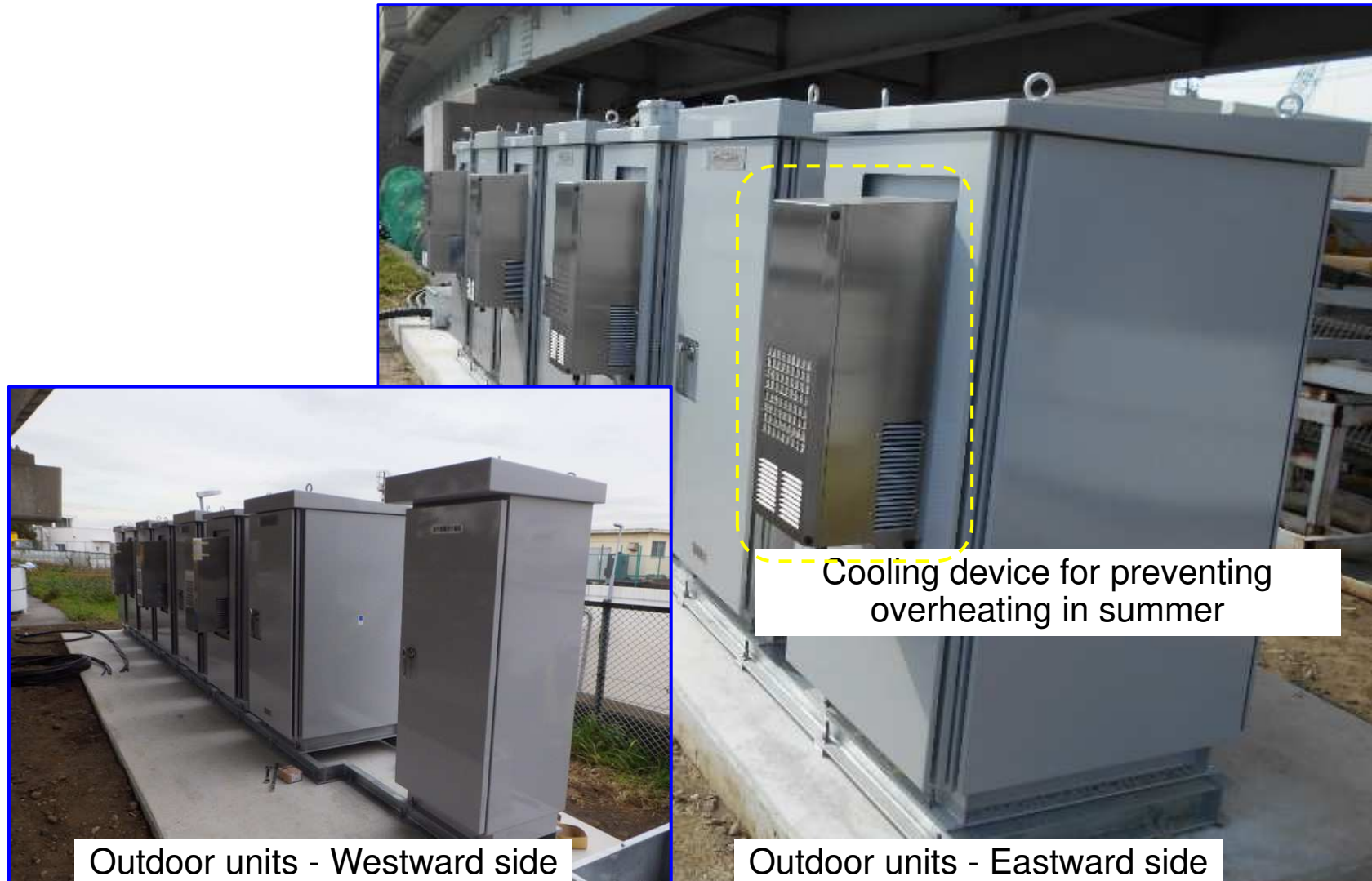
Figure 3-6 Appearance of outdoor units that house ETC gate passing support information provision management servers and roadside processing devices of individual sensor manufacturers
