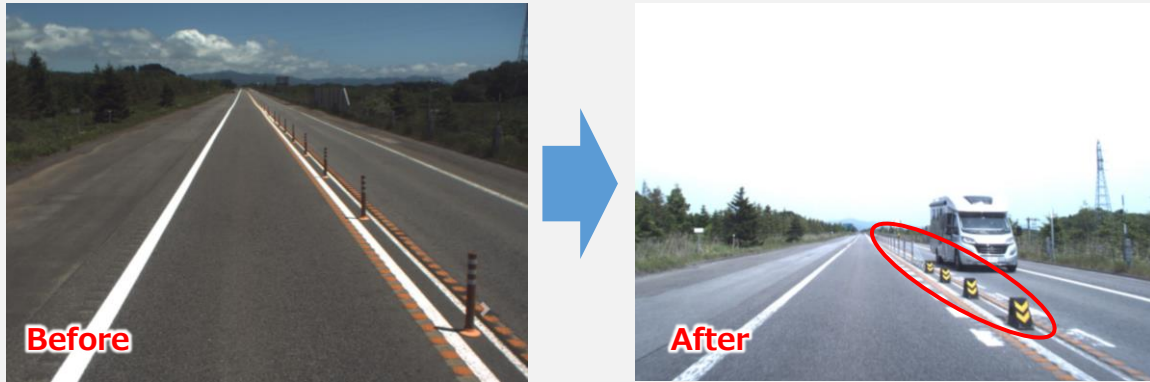
Example (1) Changes in the separation structure of a temporary two-lane section (installation of wire ropes)
